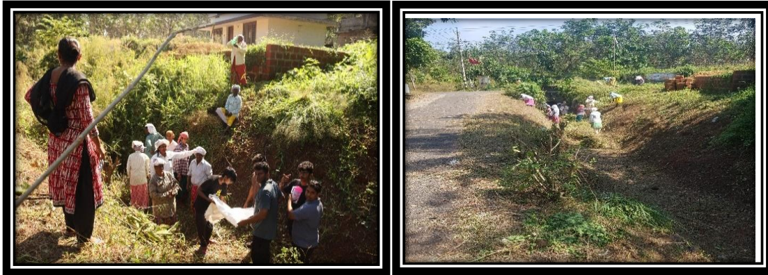
Students and MGNREGA workers of Kunnathunadu Grama panchayat cleaning the canal and nearby areas
